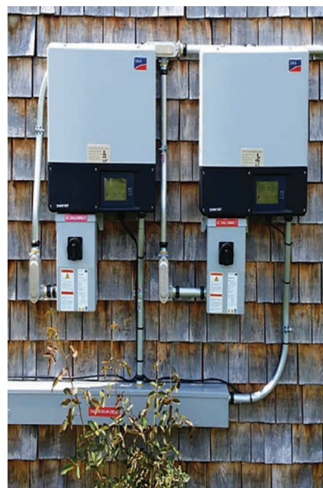
Inverters installed outside of residence
