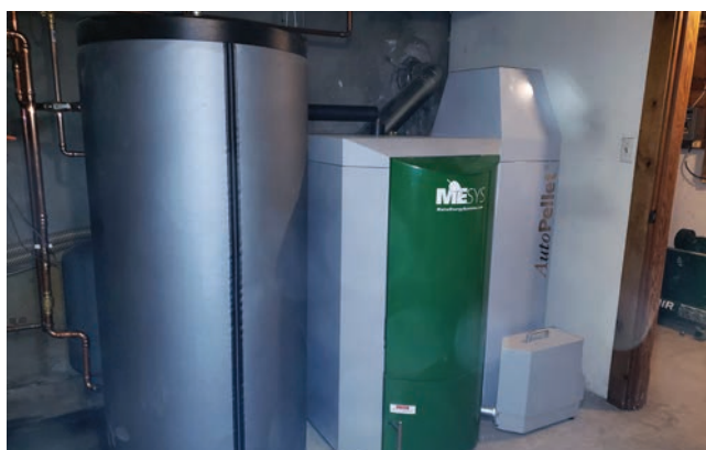
Biomass heating indoor unit
