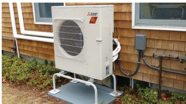
Air source heat pump external unit
